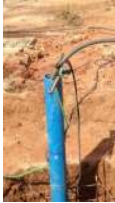
Well pumps to water tower
